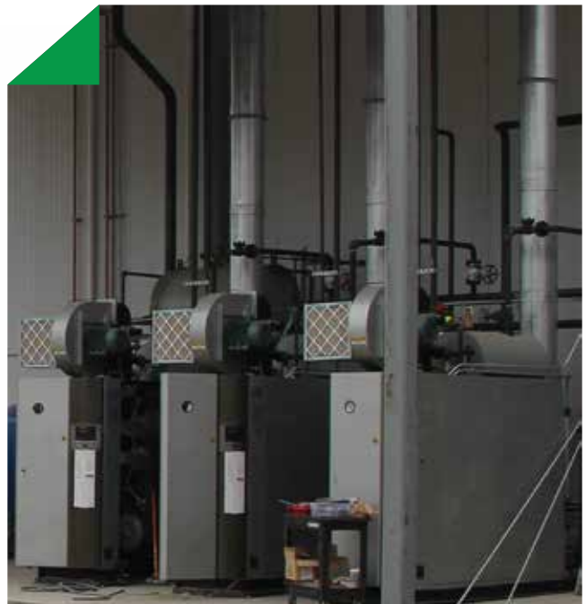
Actual boiler installation at Titan Frozen Fruit, Santa Maria, California
