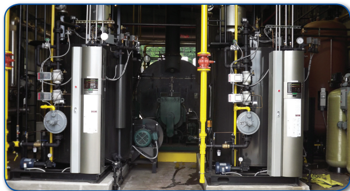
New installation of Miura EX-200 SGO dual-fuel on-demand boilers.
